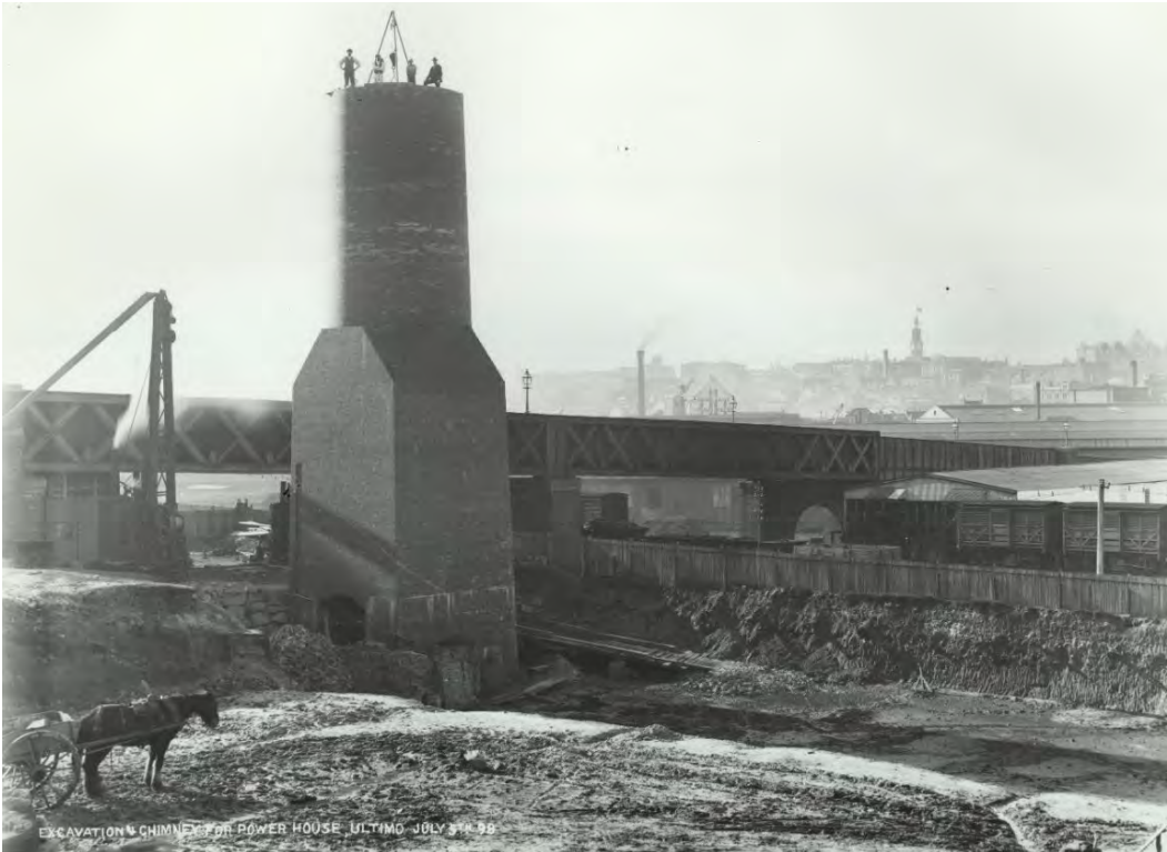
Figure 4 Power House under construction, c. 1898: view looking north-east with the William Henry Street iron bridge visible at rear
