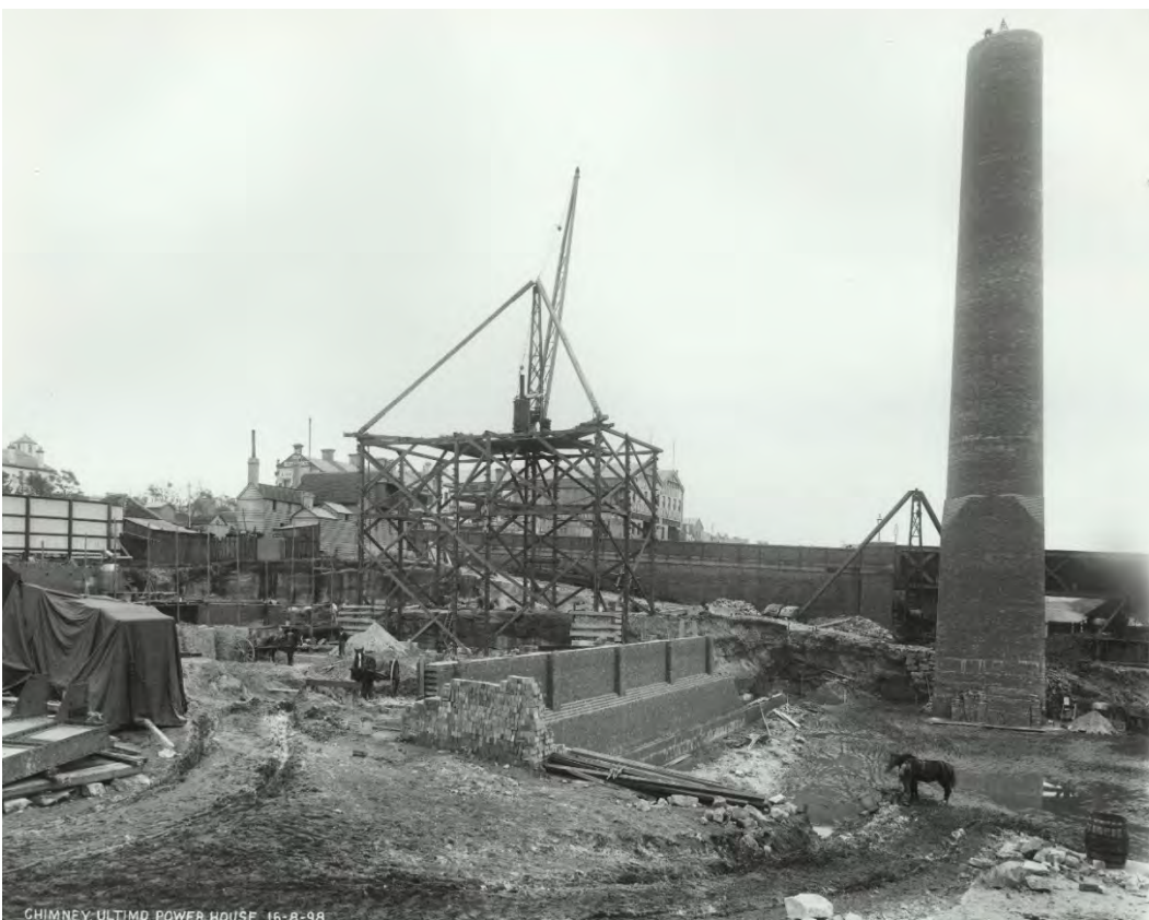
Figure 5 Power House under construction, c. 1898: view looking north to the pump room and stack
