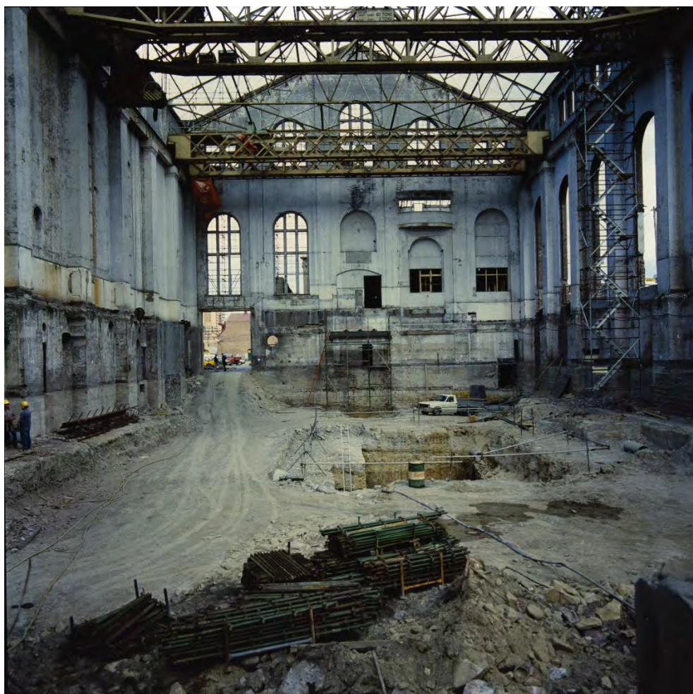
Figure 12 Interior of the Turbine Hall, facing south, during adaptive works Source: Powerhouse Museum
